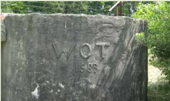
The life span of a tank can be more than 30 years if you do the maintenance
